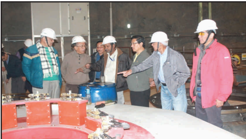
Power House of 1200 MW Teesta-III HEP
